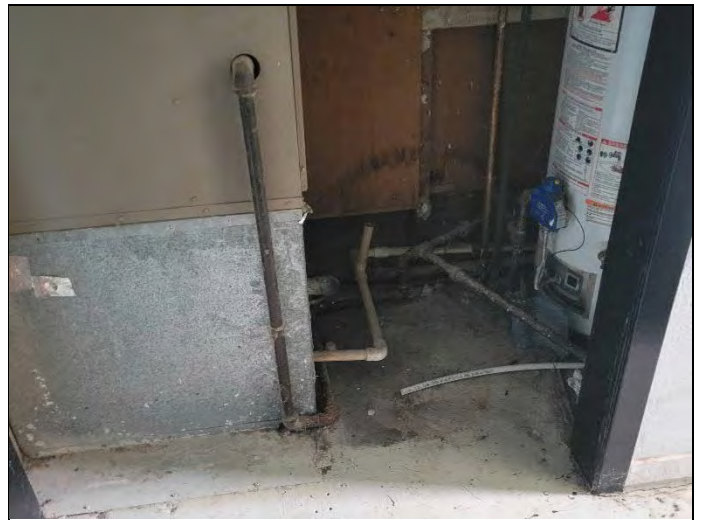
22. Subject – Interior, furnace and hot water heater
